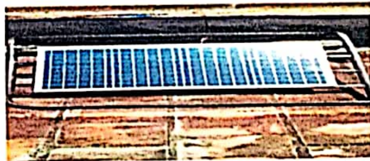
SOLAR PANEL CONNECTION
